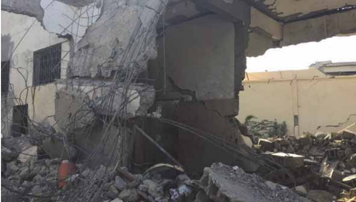
The destroyed remains of one of the wards in al-Zaydiya security directorate in Hodeida governorate. This ward and two others held at least 100 prisoners at the time of the coalition attack. Witnesses told Human Rights Watch that trucks equipped with mounted machine guns were sometimes stationed at the site. Photograph by Kristine Beckerle. © 2016 Human Rights Watch
