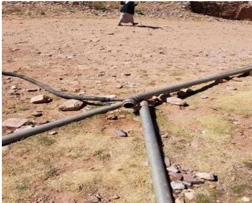
Photo: Broken pipes connecting the water network
